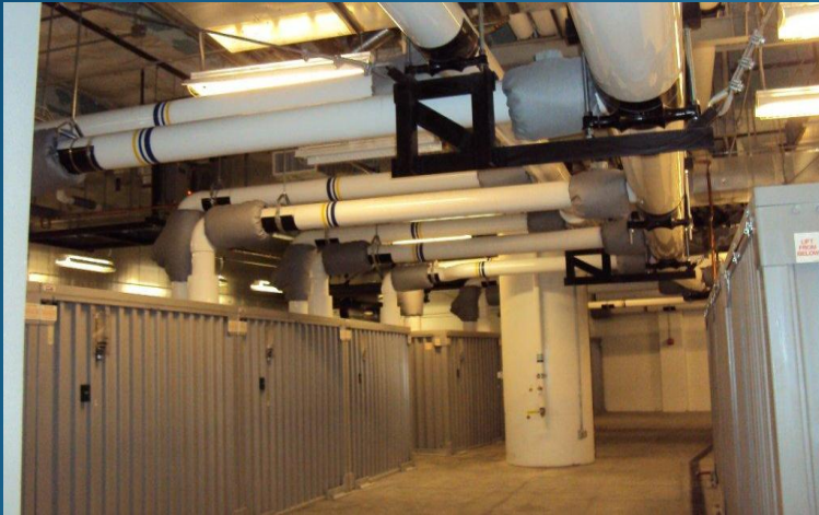
PCAP Ice Storage Tanks
